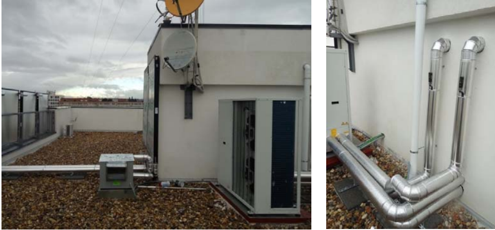
Figure 28 – Heat pump setup on the roof
