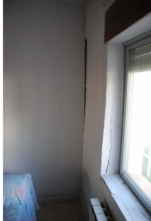
Figure 18 – Cracks inside sleeping room
