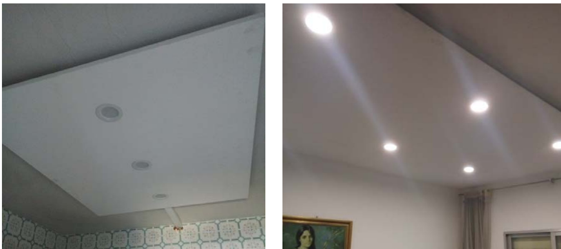
Figure 43 - Radiant panels installed
