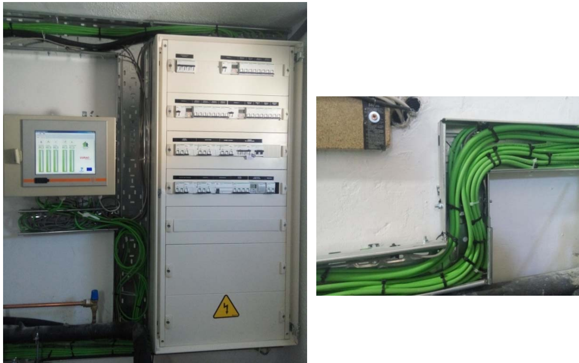
Figure 35 - Electric cabinet and Energy Manager
