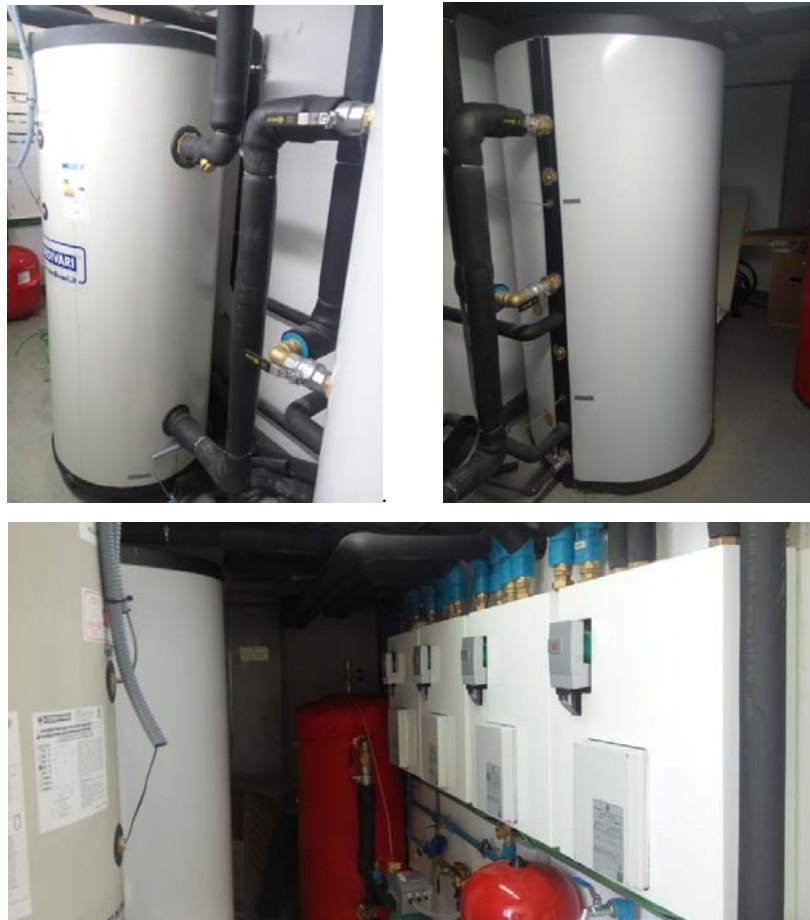
Figure 33 – thermal storage tanks and the four Energy Hubs
