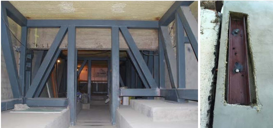
Figure 21 – Steel structure in the foundation reinforcing the existing bearing piles (left) and anchor plates (right)
