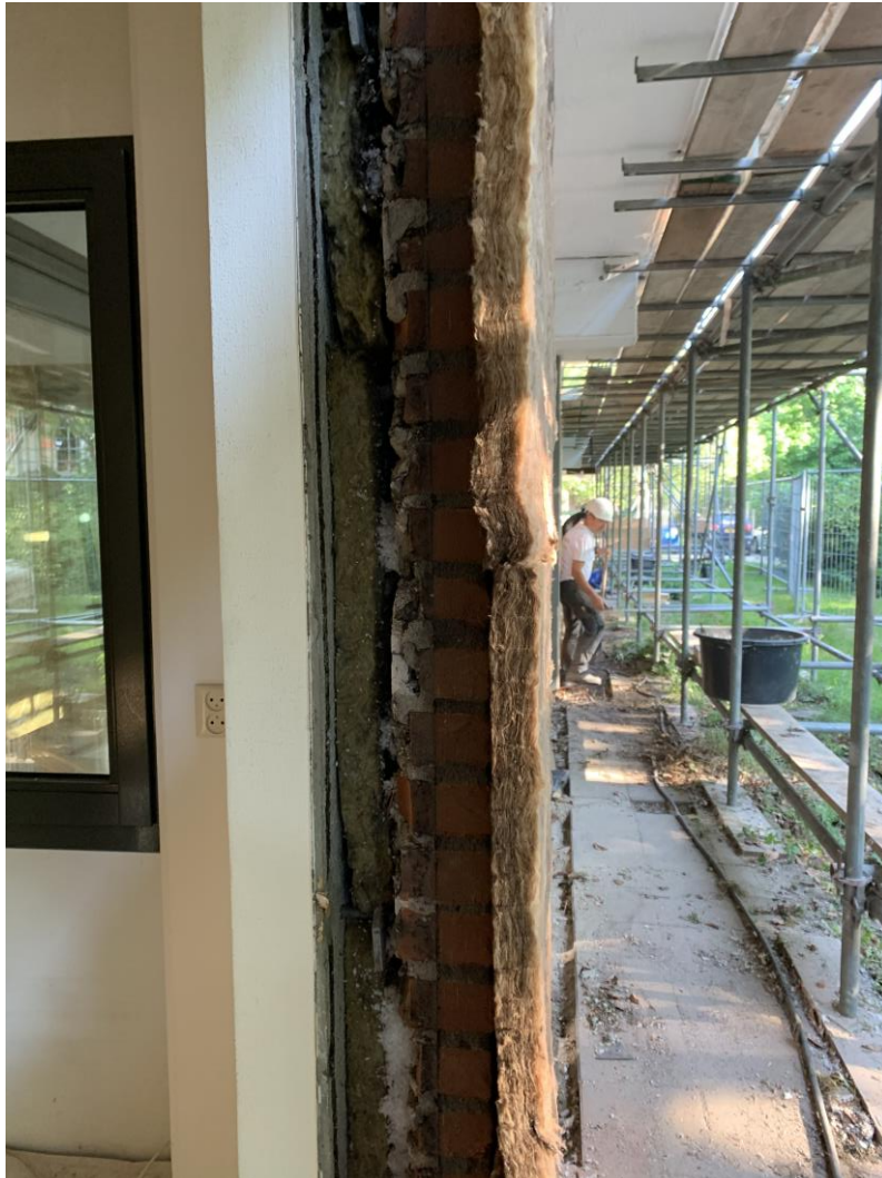
Figure 61 The existing insulated cavity has been post insulated. The exterior wall has been cladded with insulation before the prefab facades were mounted.
