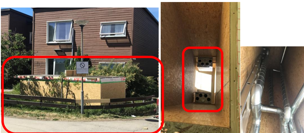
Figure 33: Prefabricated technical room/shaft in front of the building before installation (left). Technical shaft (center) with air handling units seen from above before installation of ductwork, and seen from below after installation
