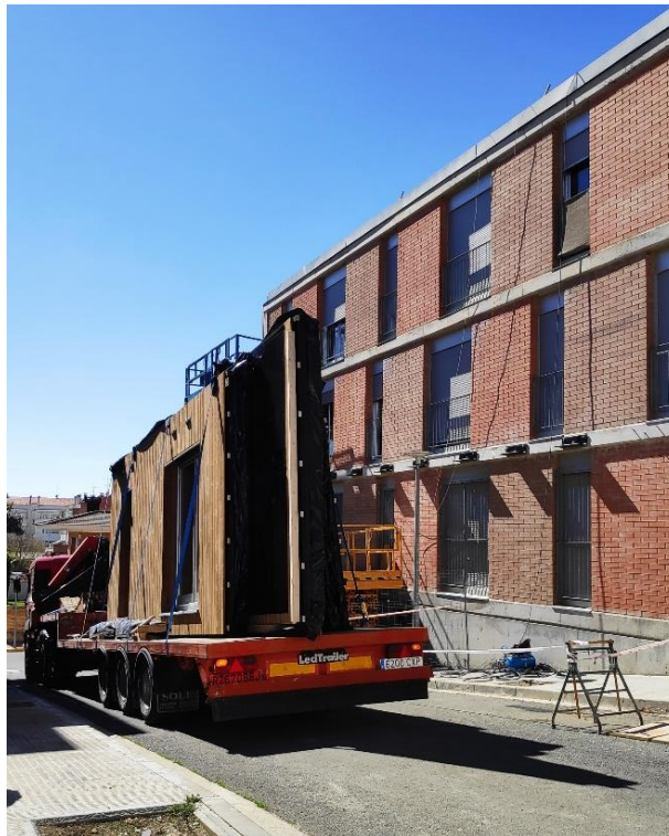
Figure 118 (left) The metal angular plates installed. (right) Installation of 1st PMF panel
