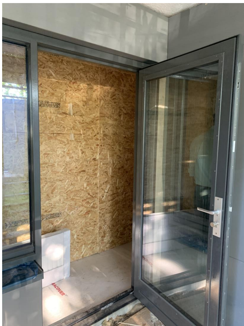
Figure 72 The temporary separation wall between the new balcony façade and the apartment.
