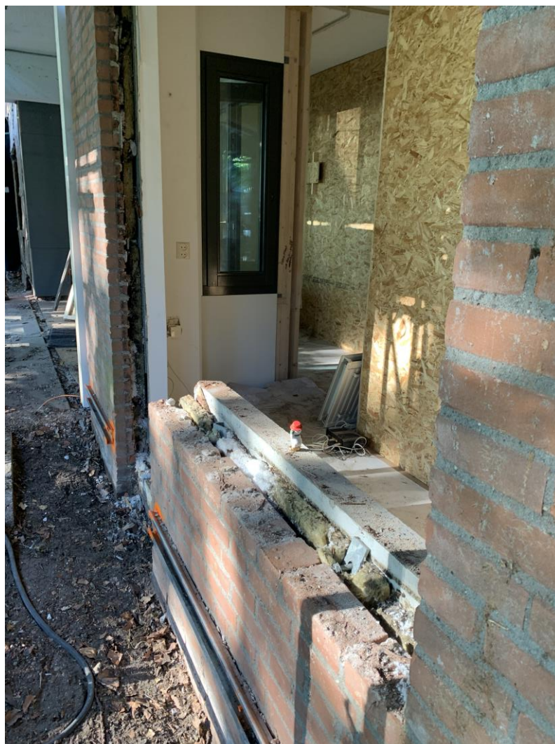
Figure 67 During two workweeks a temporary wall was constructed between the living room of the tenants and the work area for the façade renewal and prefab façade application.
