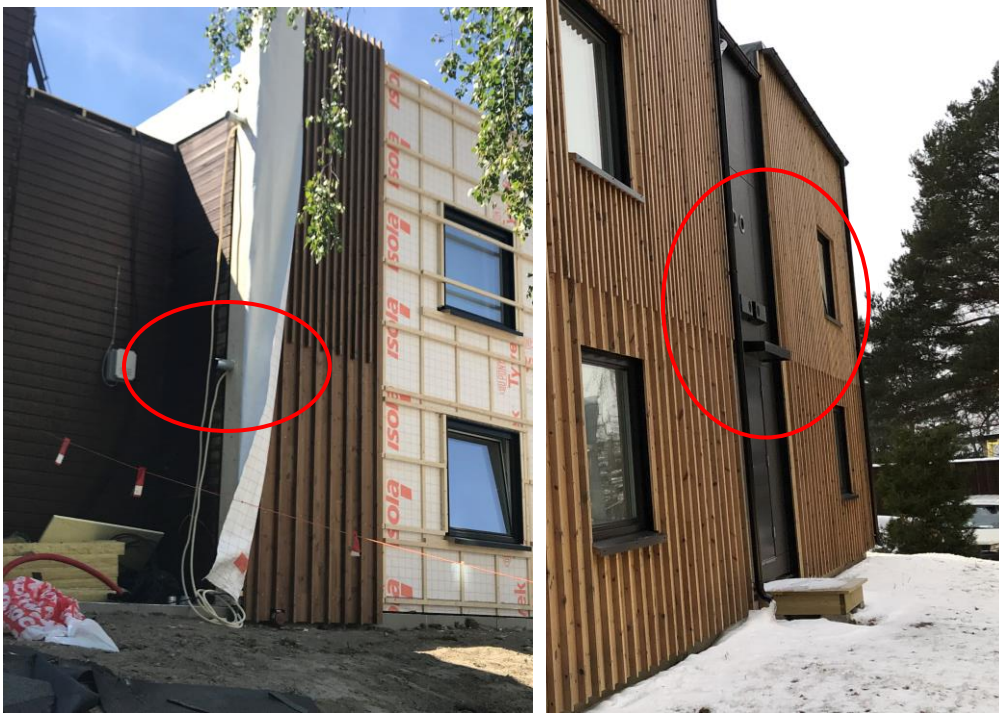
Figure 34: Ventilation duct to bedroom included in-wall element (left) and Entrance to technical room/shaft. Exhaust and inlets can be seen above the door (right).
