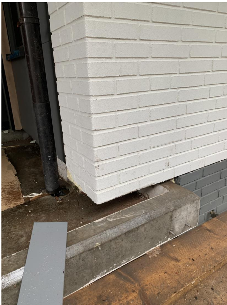
Figure 76 Detail of the connection of the prefab façade element with the existing balcony floor slab. It shows the complications of the existing structure and the precision in the design, manufacturing and mounting process, which went well without failures.
