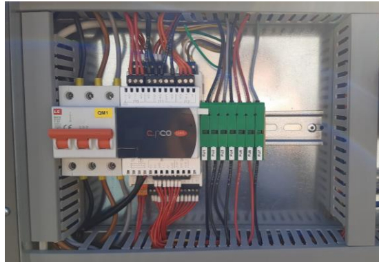
Figure 134 Heat Pump on board PLC
