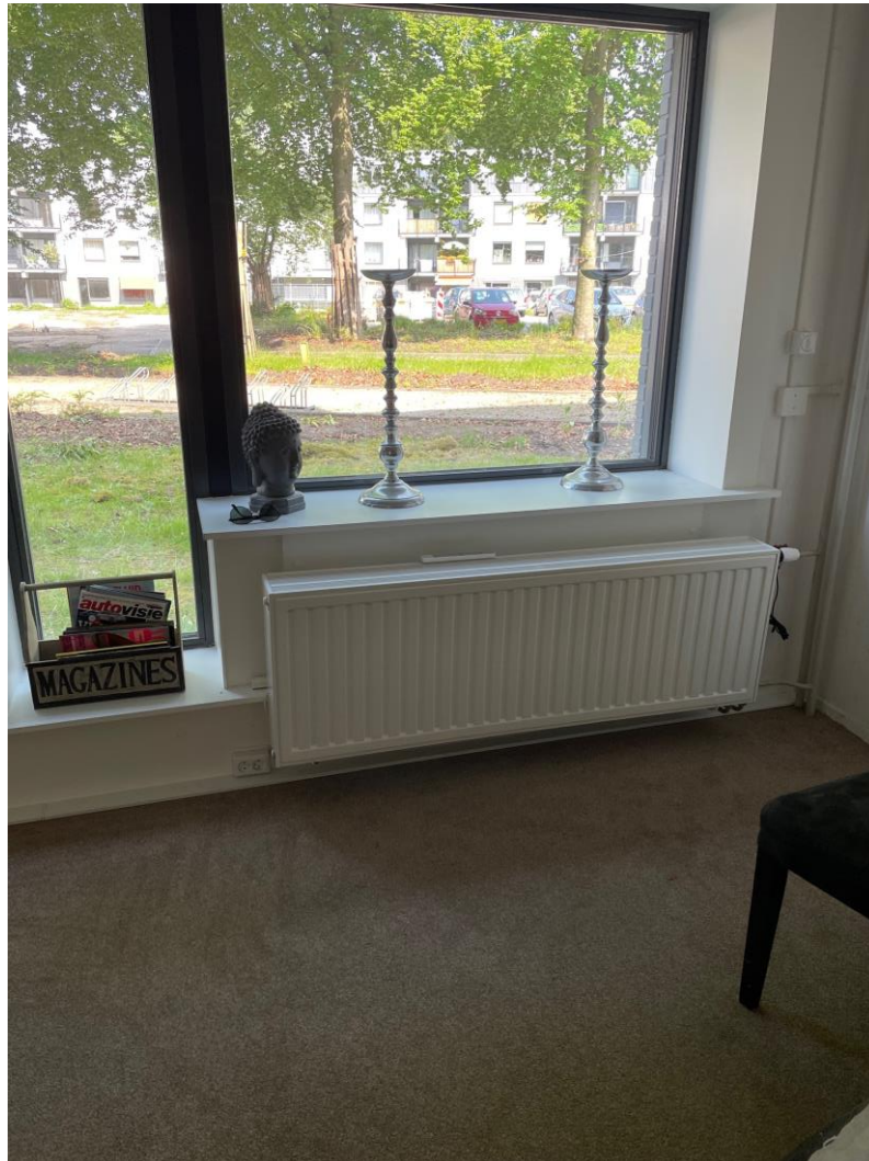
Figure 77 ClimaRad installed behind the radiator and throughout the new envelope
