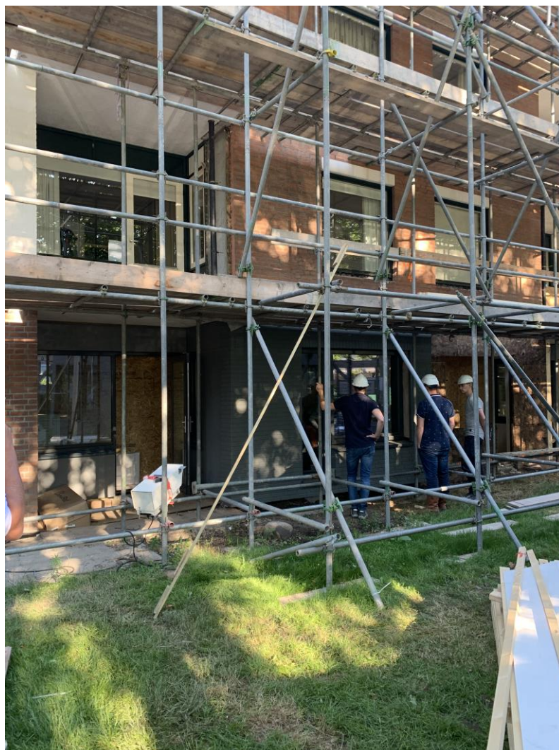
Figure 62 Scaffolding has been placed to renovate the roof and the balconies. The scaffolding has been placed on a distance to allow the mounting of the façade elements.
