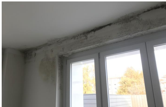
Figure 132 Presence of mold in dwelling 1 on the 1st floor
