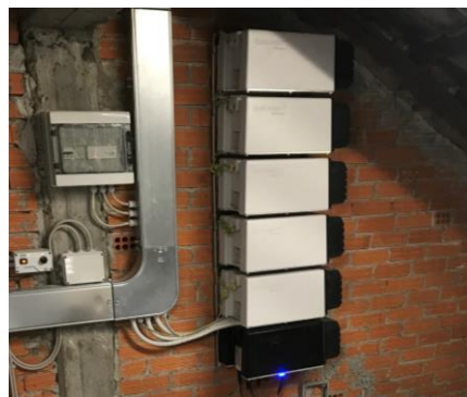
Figure 129 Electric Storage of PV system
