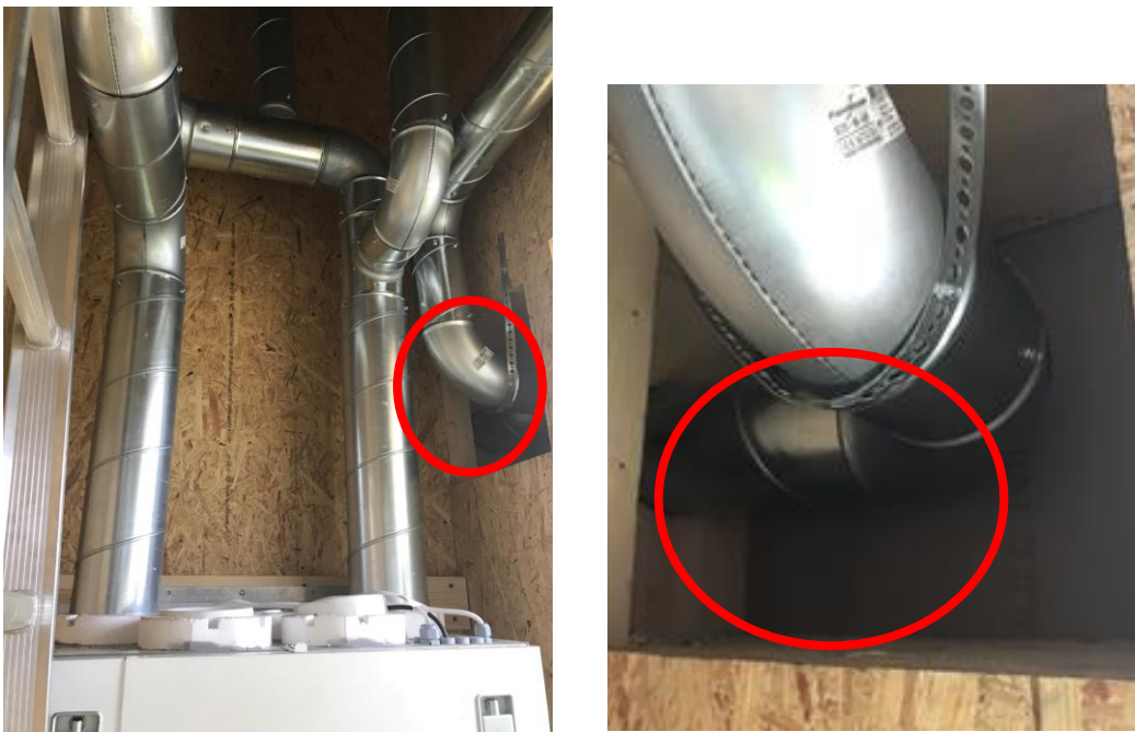
Figure 35: Ventilation ducts in the technical room / shaft. Left: Top of air handling unit is visible, right: magnified while connection to supply air duct in wall elements.
