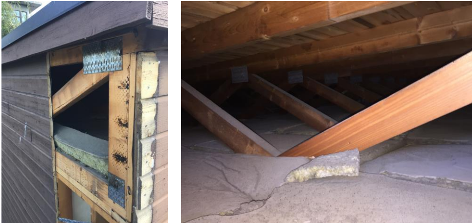
Figure 11: The façade was opened, and the state of the load-bearing constructions was analysed. The aerated concrete bricks are clearly visible. The outer wall does not seem to have major damages or faults. The state analysis shows that the construction is in good shape, with no sign of moisture damages.
