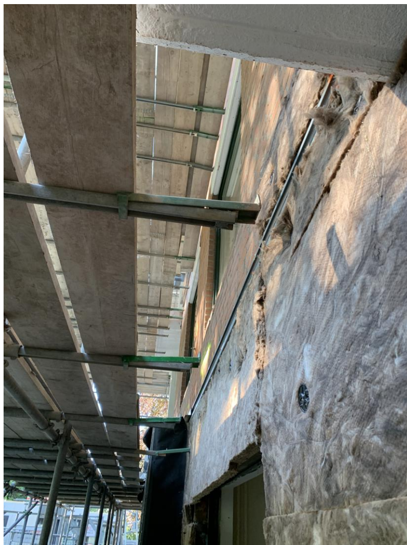
Figure 66 Hilti railing system is mounted on the exterior façade. This method has been successfully used in previous project by Prefabfabriek Culemborg.
