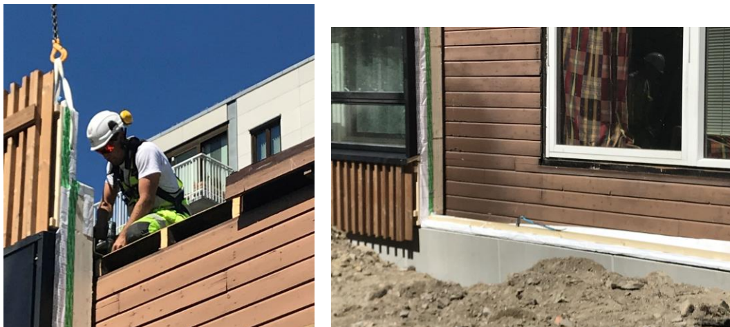
Figure 30: Details – securing of wall element and wall element mounting on new foundation
