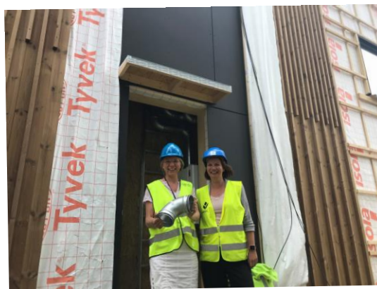
Figure 46: Kari Thunshelle from SINTEF (left) and Vera Lukina (right) outside the technical room inspecting the installation of the ventilation system.
