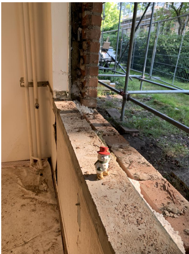
Figure 79 The existing radiator has been dismantled to be replaced with the Climarad decentralized heat recovery radiator.
