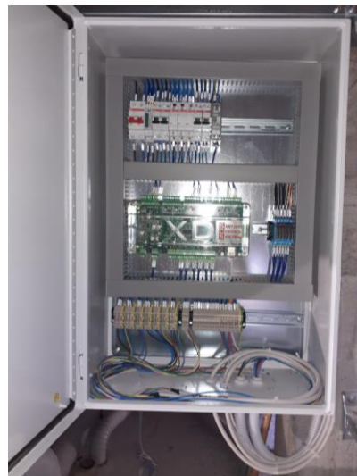
Figure 142 HVAC Electrical panel of a dwelling
