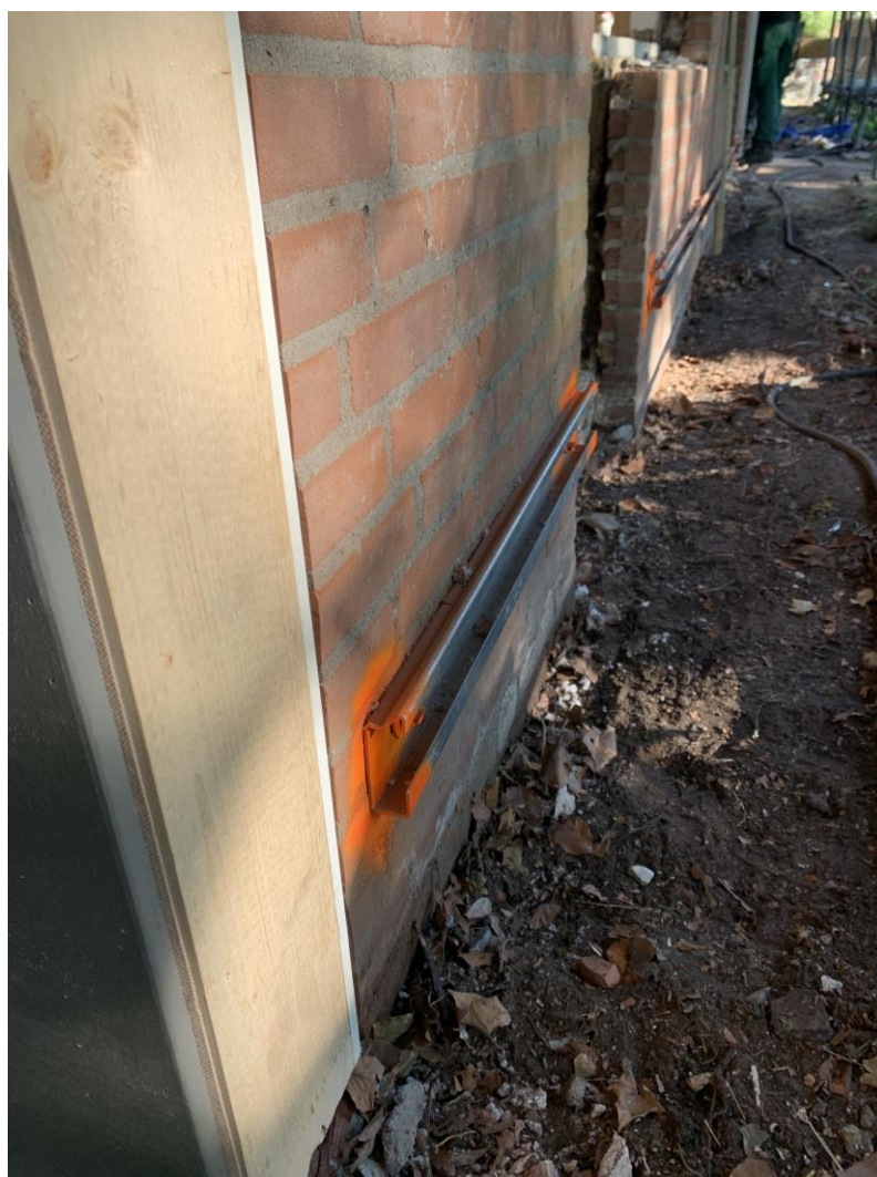
Figure 65 The first Hilti rail mounted on the exterior of the cavity wall construction.
