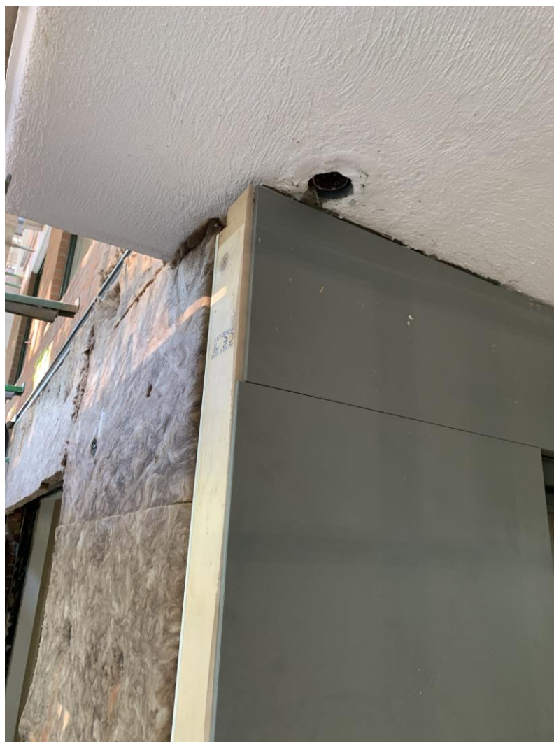
Figure 71 The width of the façade element adjacent to the balcony has been designed to leave space for the rainwater gutter.
