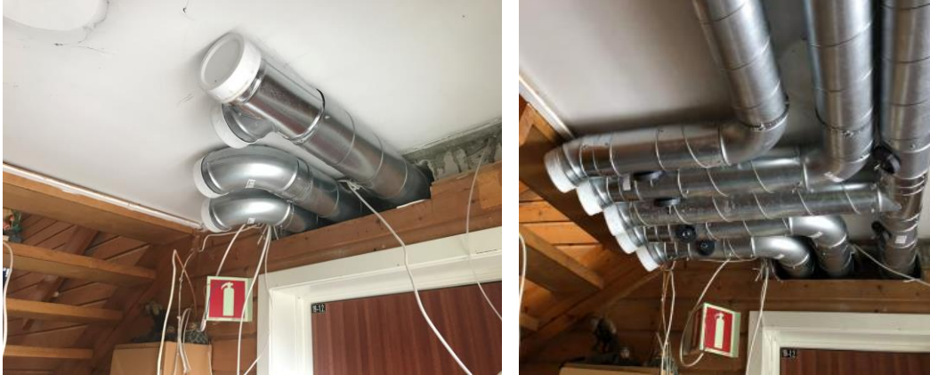
Figure 39: Ductwork from entrance in apartment to main entrance, to be connected to ducts underneath the stairway
