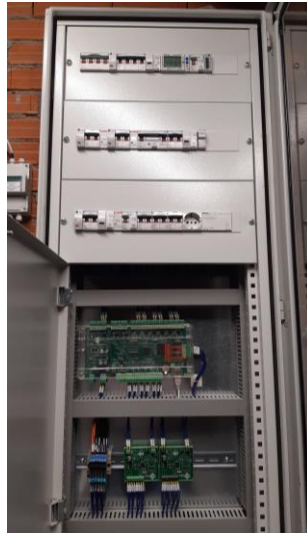
Figure 141 The main switchboard
