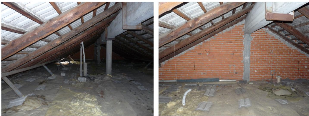
Figure 124 Attic situation before 2020 interventions, with the damaged mineral wool insulation
