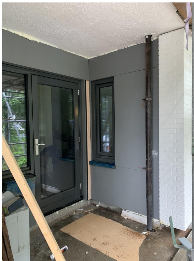
Figure 73 Installed prefab façade elements around the balcony. Afterwards thermal bridge insulation has been added on the floor and ceiling of the balconies.
