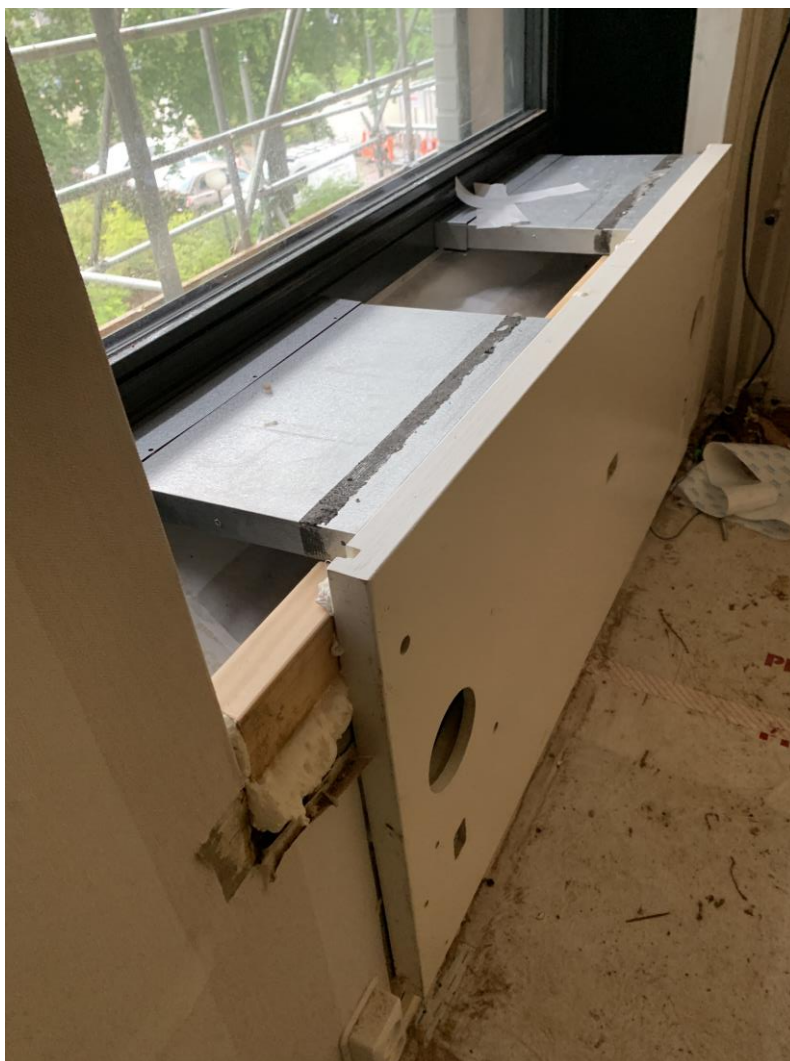
Figure 81 Ducts connecting the façade to the interior (supply and exhaust air)
