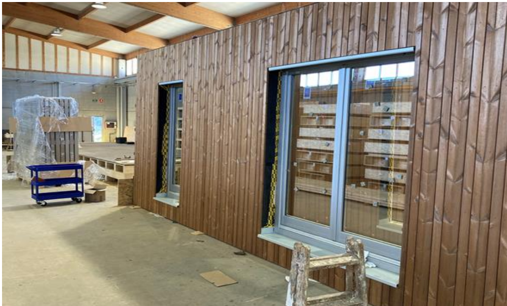
Figure 115 PMF façade panel from 1st floor almost finished and stored in the Workshop.
