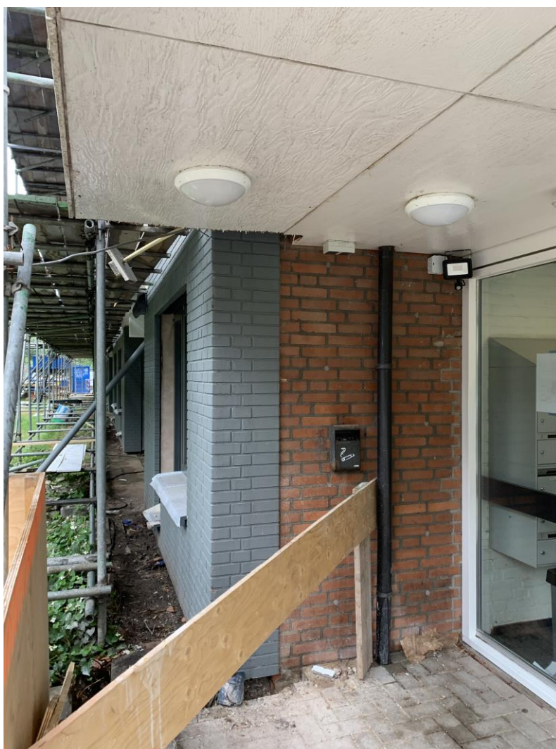
Figure 74 Connection of prefabricated façade and cavity wall façade near the building entrance
