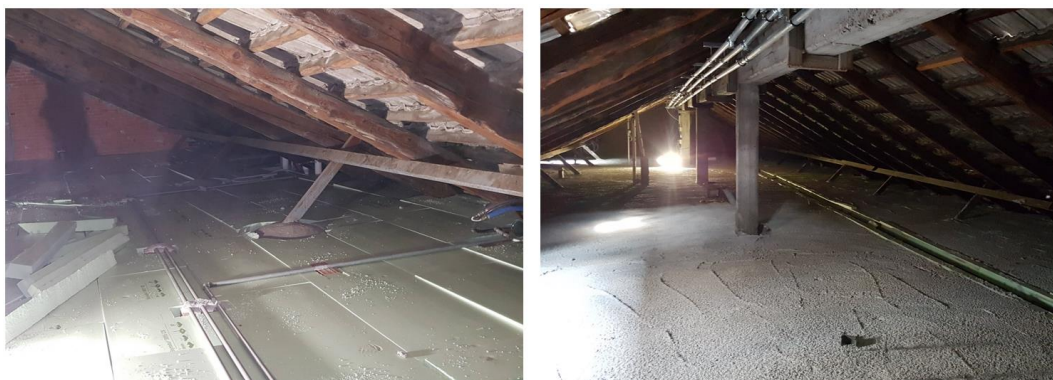
Figure 125 Attic during EPS coating (on the left) and the final result with light concrete slab (on right)
