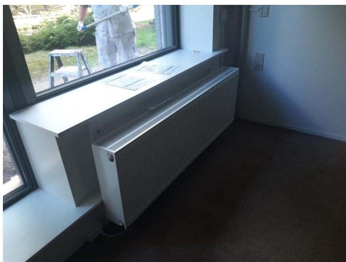
Figure 82 The completed decentralized ventilation radiator
