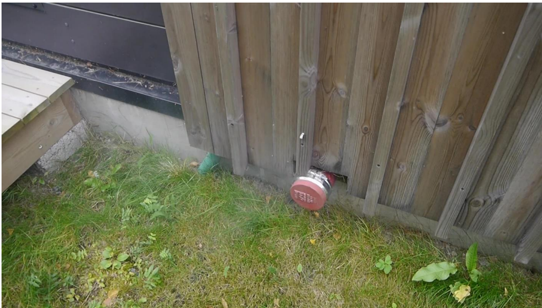
Figure 44: Smoke in the passage for downpipes, before sealing
