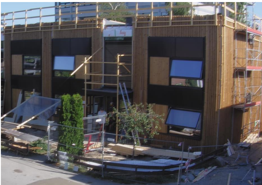
Figure 25: Hagerudsenteret 17-19 during renovation June 2018. Half of the building was renovated at a time. The upper picture right side show existing building with dismantled protruding parts of roof and windows.
