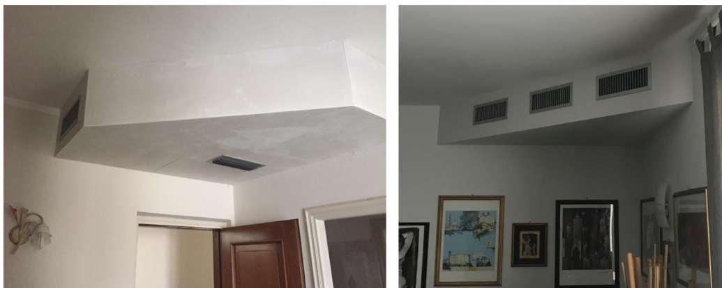
Figure 127 New fan coils hidden in the false ceiling
