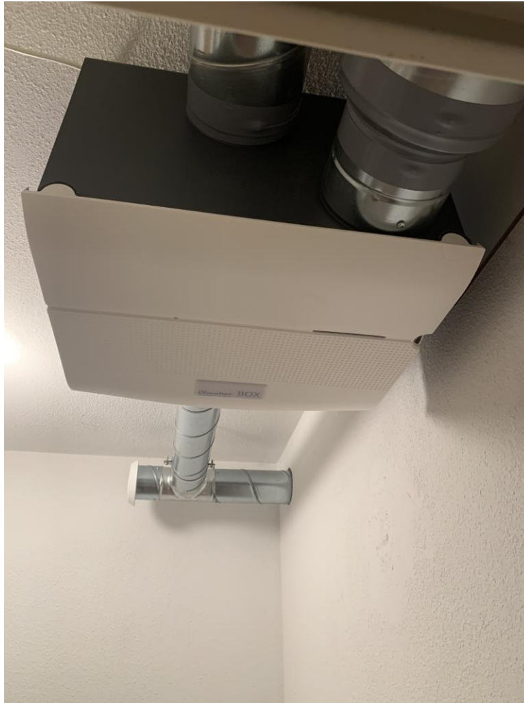
Figure 83 Climarad exhaust fan for bathroom, toilet and kitchen in the 4RinEU demo-apartments.
